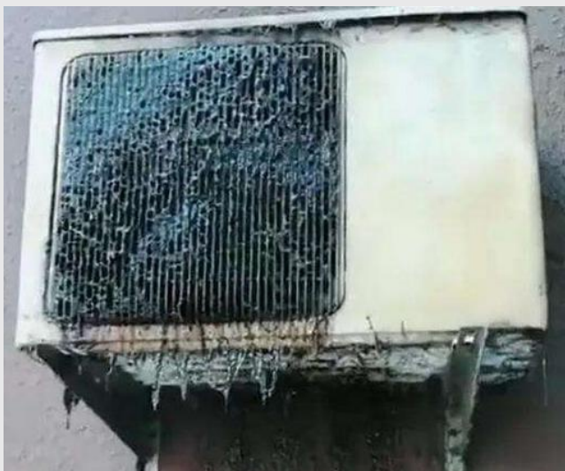
ODU is too dirty 外机脏堵
