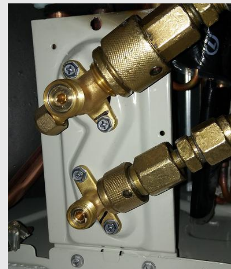
Stop valve fully open
